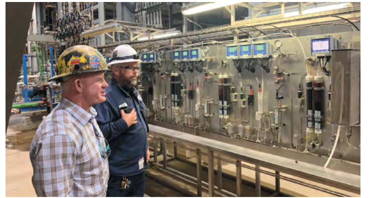
Second District International Vice President Mike Monahan, left, inside the Salem Harbor Power Station with Lawrence, Mass., Local 326 steward Geoffrey Winn Jr., an operations and maintenance technician.
